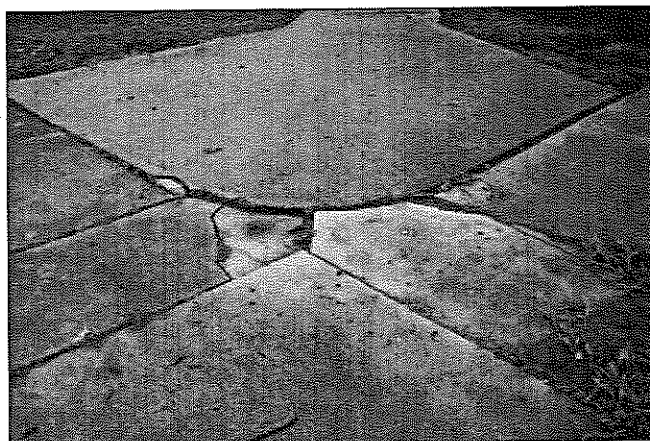
A sidewalk in need of repair.
